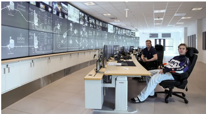
Fig. 4. Illustration of the new control room at Elkem Bremanger (Teknisk Ukeblad)
